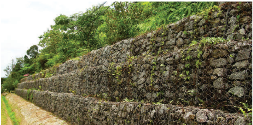
Gambar 5.11: Benteng gabion menahan tebing daripada terhakis/runtuh.
